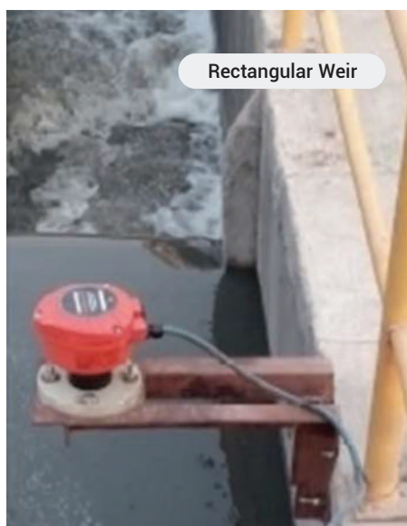
Effluent Treatment Plant
